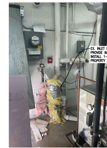
ISD GEN EDUCATION BUILDING PIPING FROM WELL
